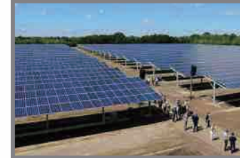
Solar Power Plant Power: 2MW
