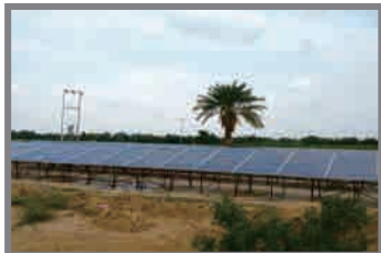
Solar Pumping System Power: 54KW
