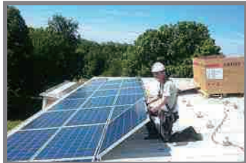
SAKO Solar Installation Middle East Countries
