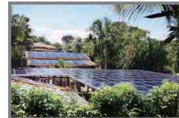
Solar Power System Salvador Pousada Hotel
