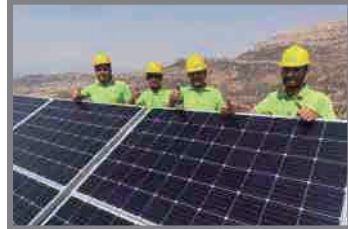
SAKO Solar Installation Middle East Countries
