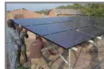
Solar System Installation For Hospital Organization
