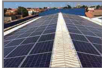
Solar Building Roof Power: 100KW
